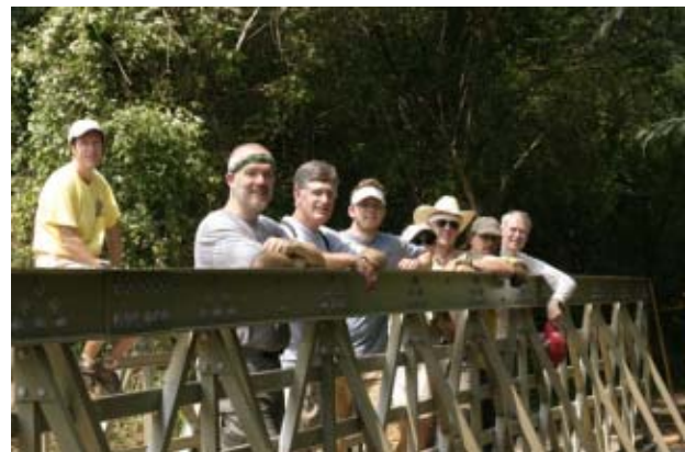
Bridge Work Crew - some of the folks who worked to put the bridge in place.
